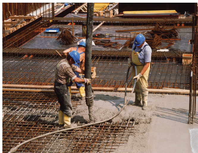
Image C9.06 Construction workers using a pump to lay concrete around a mesh of metal rods. The rods will strengthen this reinforced concrete.
